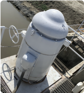
Canal Lift Pumps
