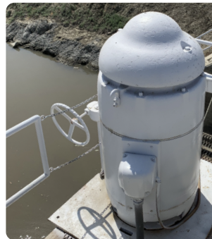
Canal Lift Pumps
