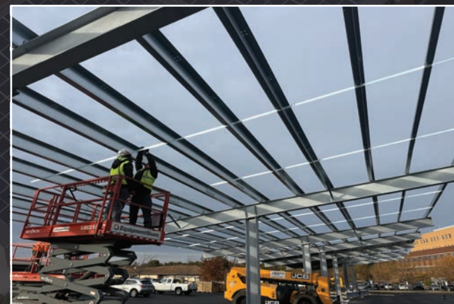
Hospital Carport: 500KW
